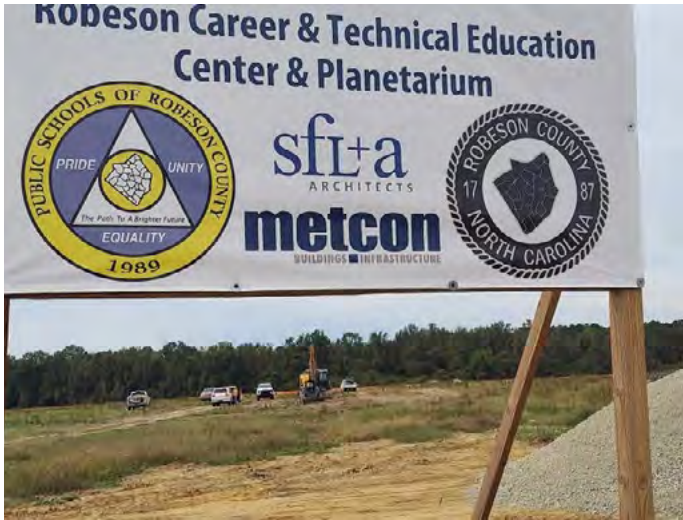
Here is an image of the lot we're building on, in the initial stages of being leveled.
