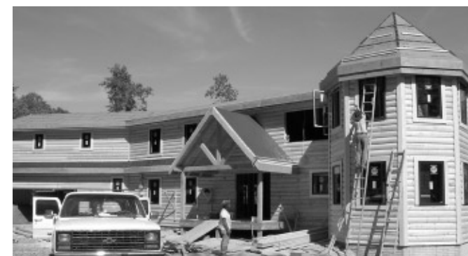
Work continues on our home. The windows, siding, entrance-way porch, and first-floor false eave are installed. A. Thanz
